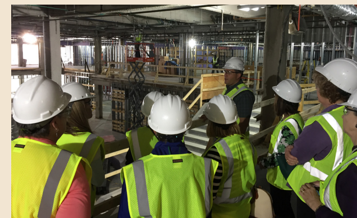
ABOVE: This past June, several EMMC Auxiliary members took a hardhat tour for a close look at the construction site at EMMC, including the new home for EMMC's NICU which the auxiliary is currently raising funds for.
